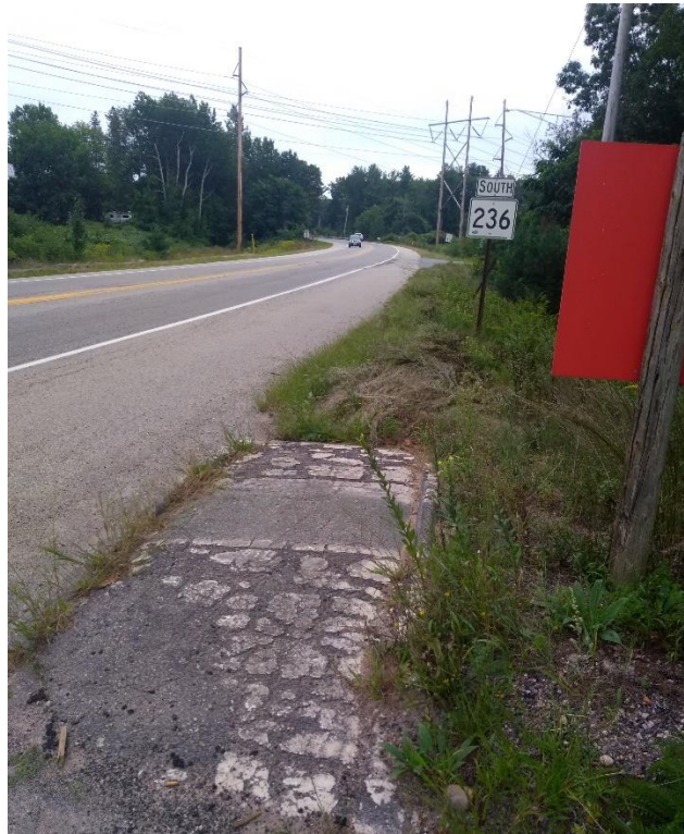
Figure 38. Route 236 looking south toward Heron Cove Rd. The project proposes to build a sidepath along this stretch, restoring and widening the deteriorated sidewalk and creating a new link in the Eastern Trail and East Coast Greenway, as part of a larger intersection improvement project recommended in the Route 236 Corridor Study.
