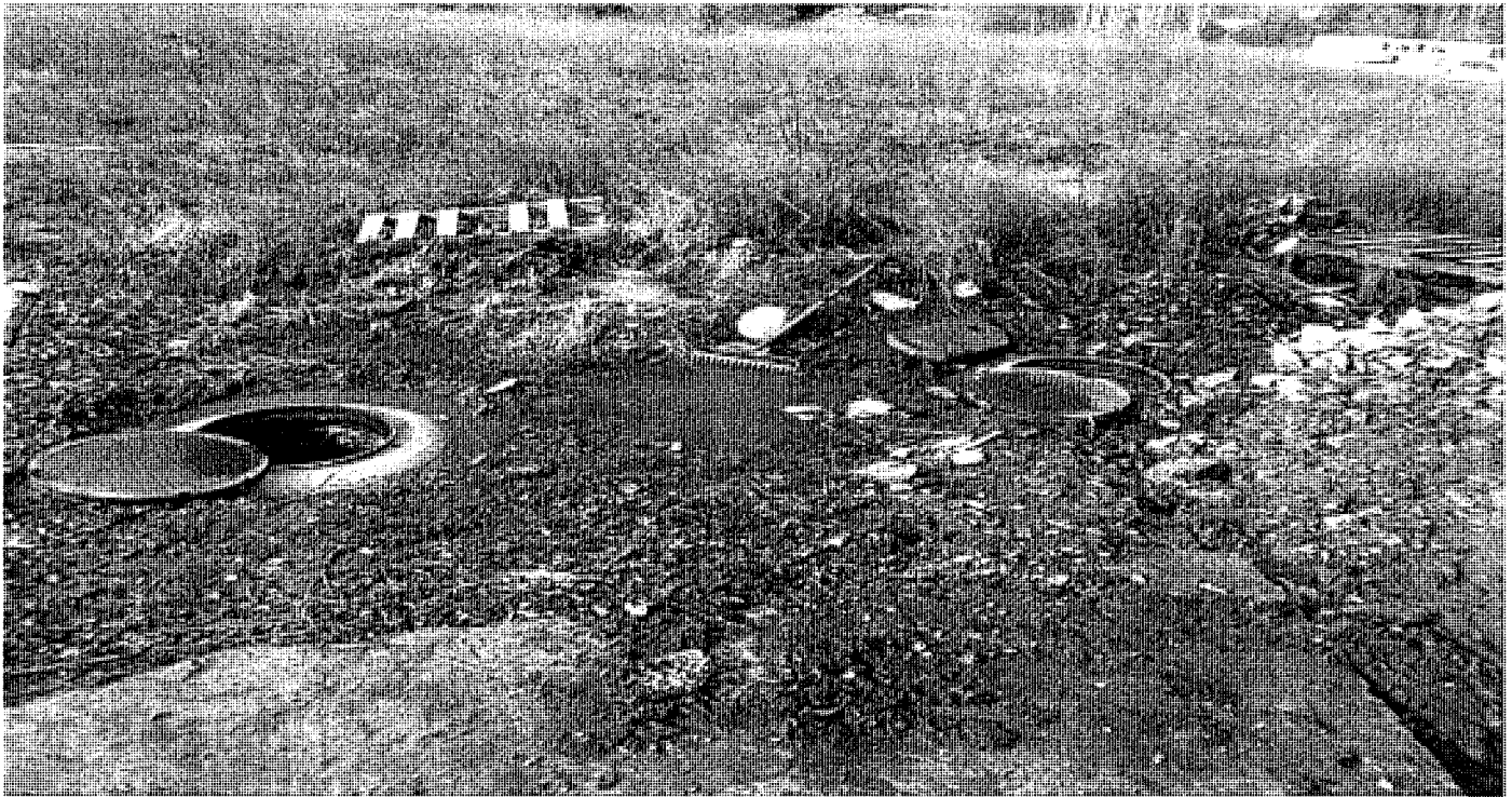
Brick-and-mortar risers at the septic tank center and at the pump chamber.
